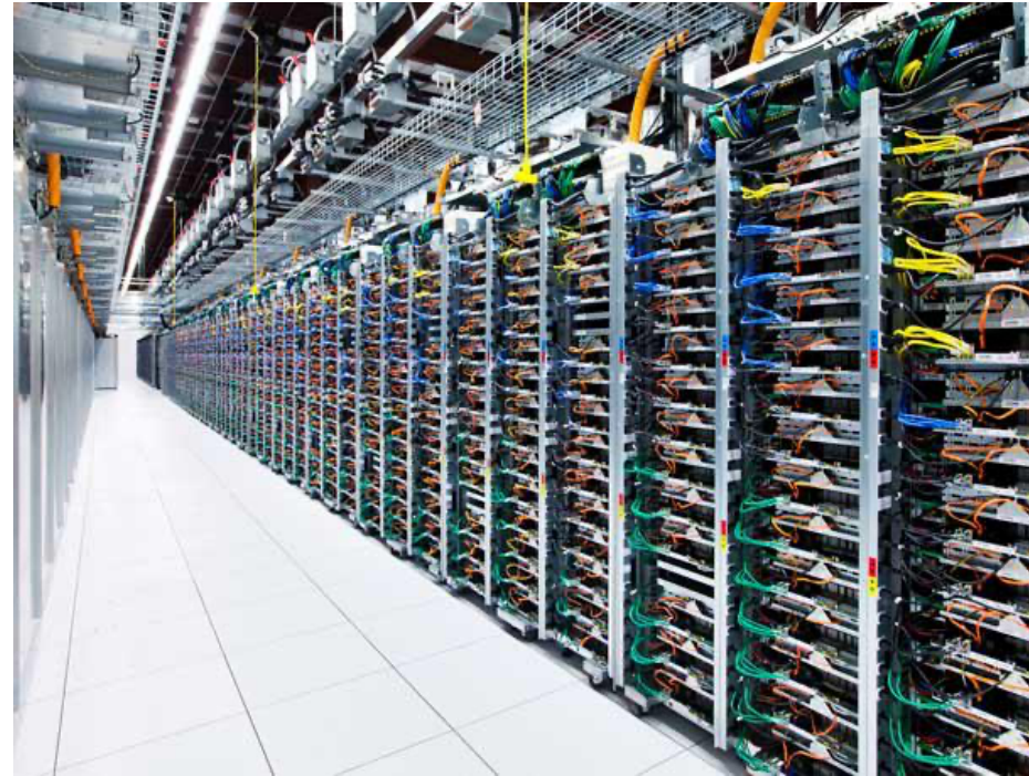
Up to millions of servers in a typical data center
